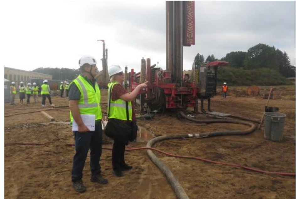
Agawam High School, Agawam – MSBA Tour of Geothermal Well Drilling Site (October 2025)
